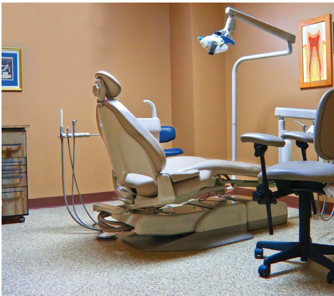
The FLEXMAR polyaspartic coating was applied directly to the existing VCT flooring, reducing overall application time and labor costs.
